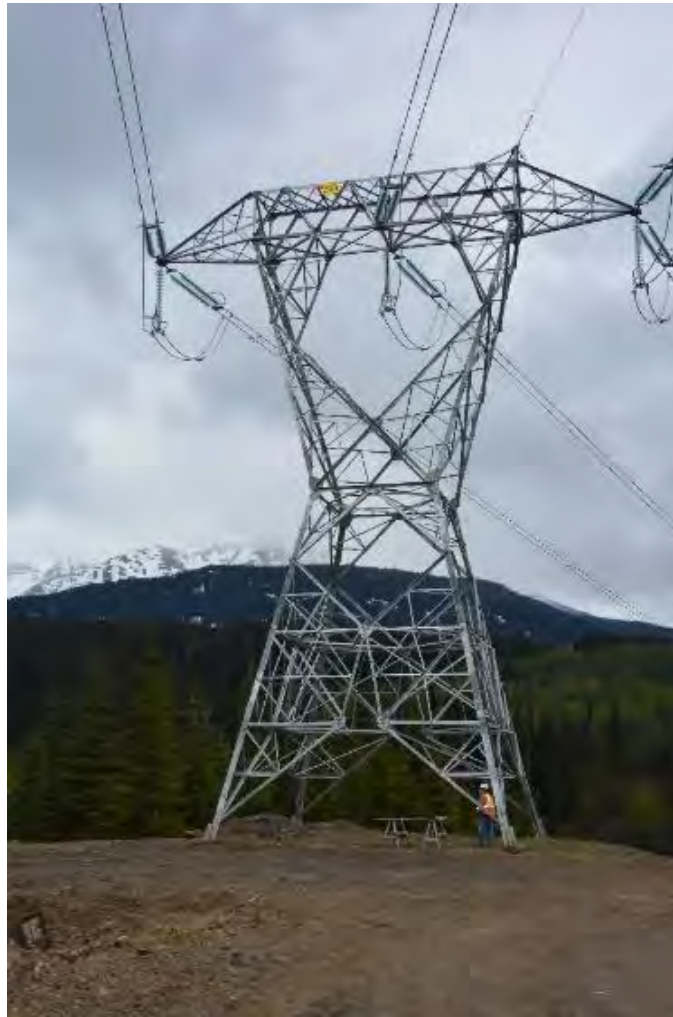
Figure 18-25: Typical 287 kV Self-Supporting Tower
